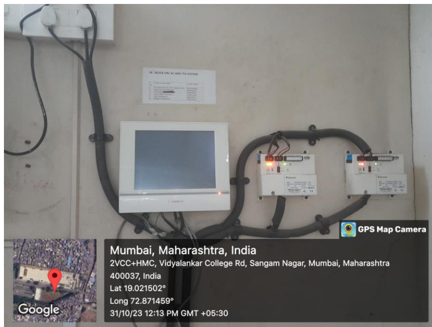
Figure 2.2. Intelligent Temperature Machine (ITM) unit, Basement, M-block, VIT
