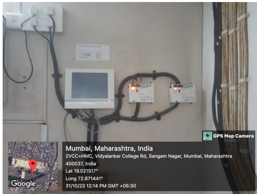
Figure 2.1. Intelligent Temperature Machine (ITM) unit, Basement, M-block, VIT
